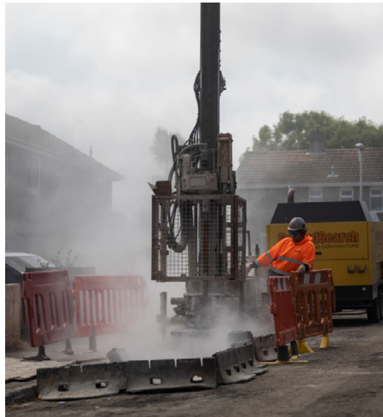
Photo credit: Kensa Utilities
